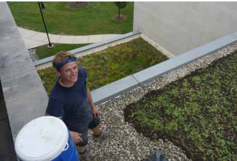
Andrew after spreading the last of the Sedum cuttings. Seem below is one of the green roofs we installed the previous summer.
